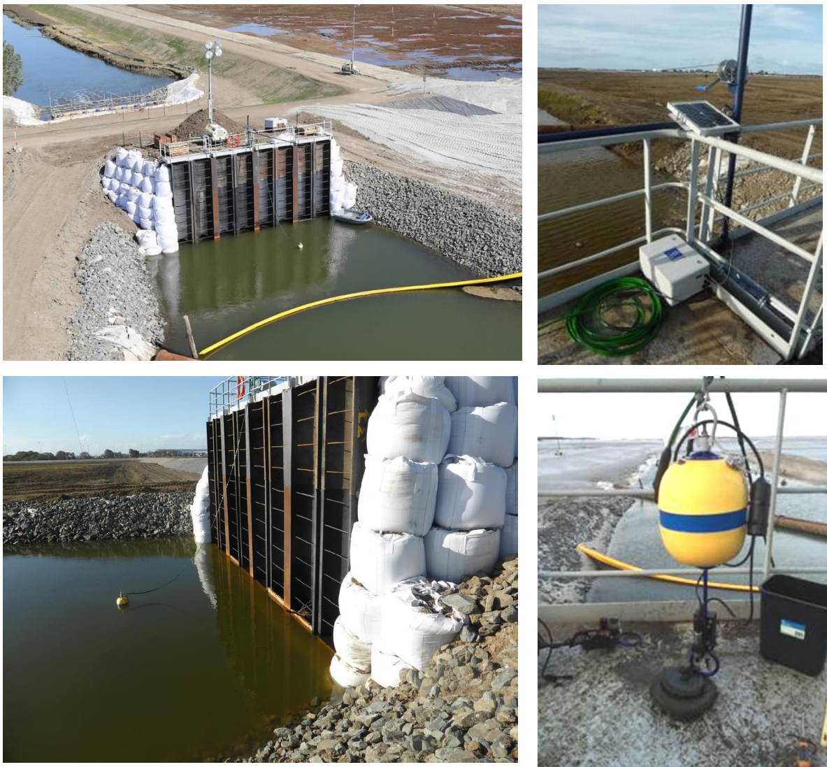
Figure 3-18: Water box continuous turbidity monitoring installation.
