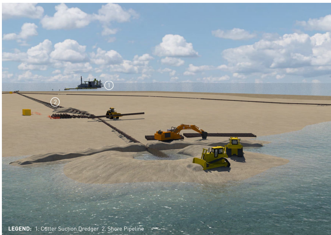
Figure 7-1: For discharge onshore, the CSD (1) connects to a discharge pipeline that consists of floating, submerged and onshore pipes (2)
