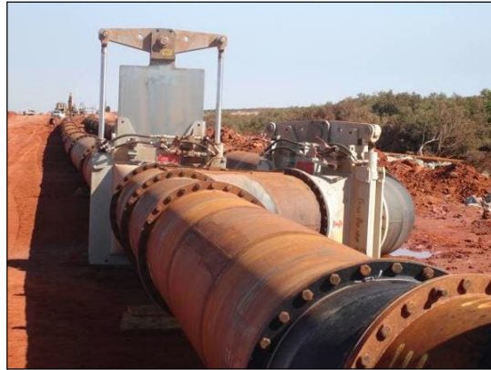
Figure 6-19: Y connection in the pipeline with hydraulic valve operation
