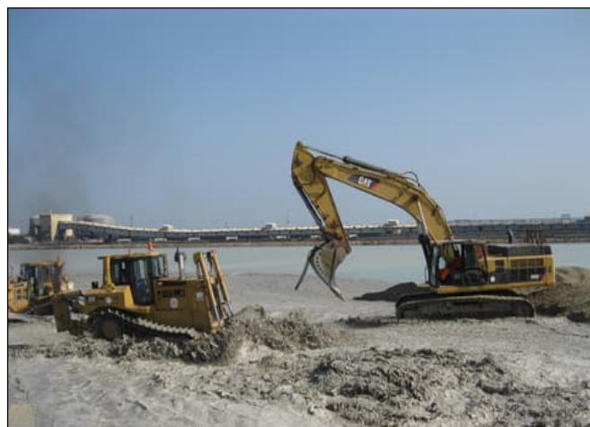
Figure 6-8: Dry Equipment on the discharging Area
