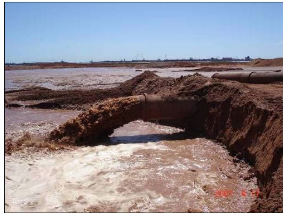
Figure 6-16: Outflow of material in discharge area
